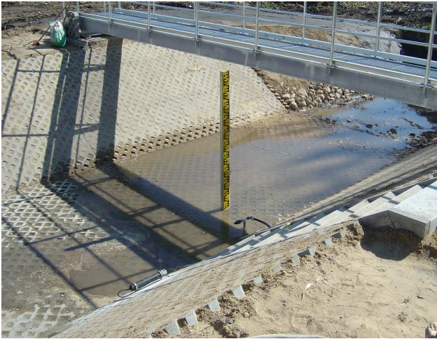
Trapezoid construction and mounting around the measurement-cross-section (Picture: StAUN Schwerin)
