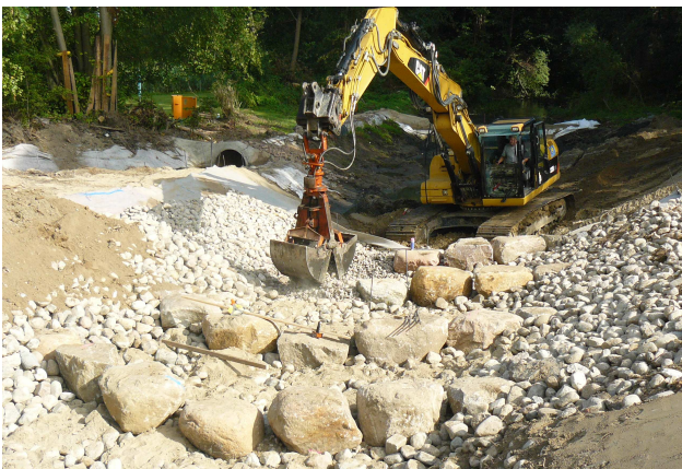
Construction of the rock ramp with a shovel with a long grab
